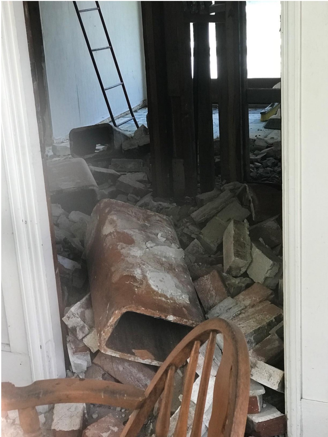
Exhibit 4-A: Initial investigation and stop work order posted. Demolition of walls and chimney, seen in plain view through clear glazed front entry doorway. Photo taken 10/12/2020.
