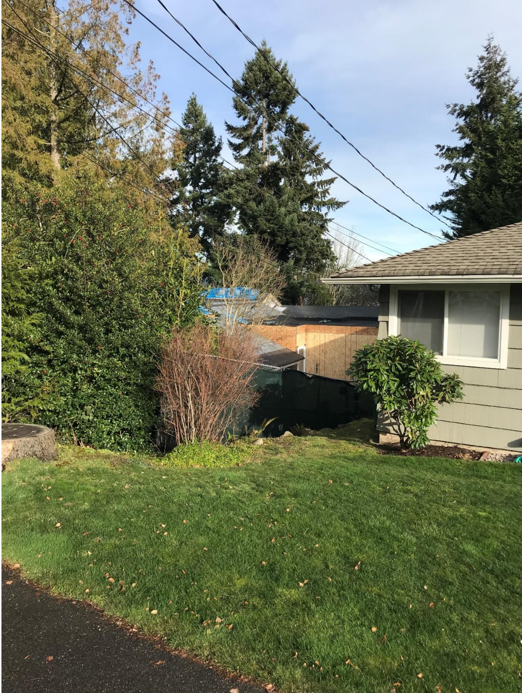
Exhibit C: Continuance of work in violation of SWO; Unpermitted addition. 01/27/2021
